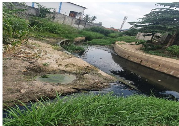
Discharge of industrial effluent in Food Security one Stormwater Drain in Ilala
