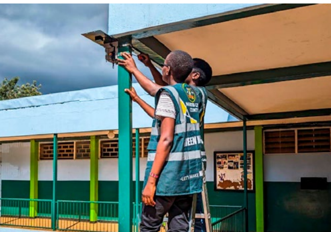
Air quality measurement devices are being installed at Kenyatta University Primary School in Nairobi.
